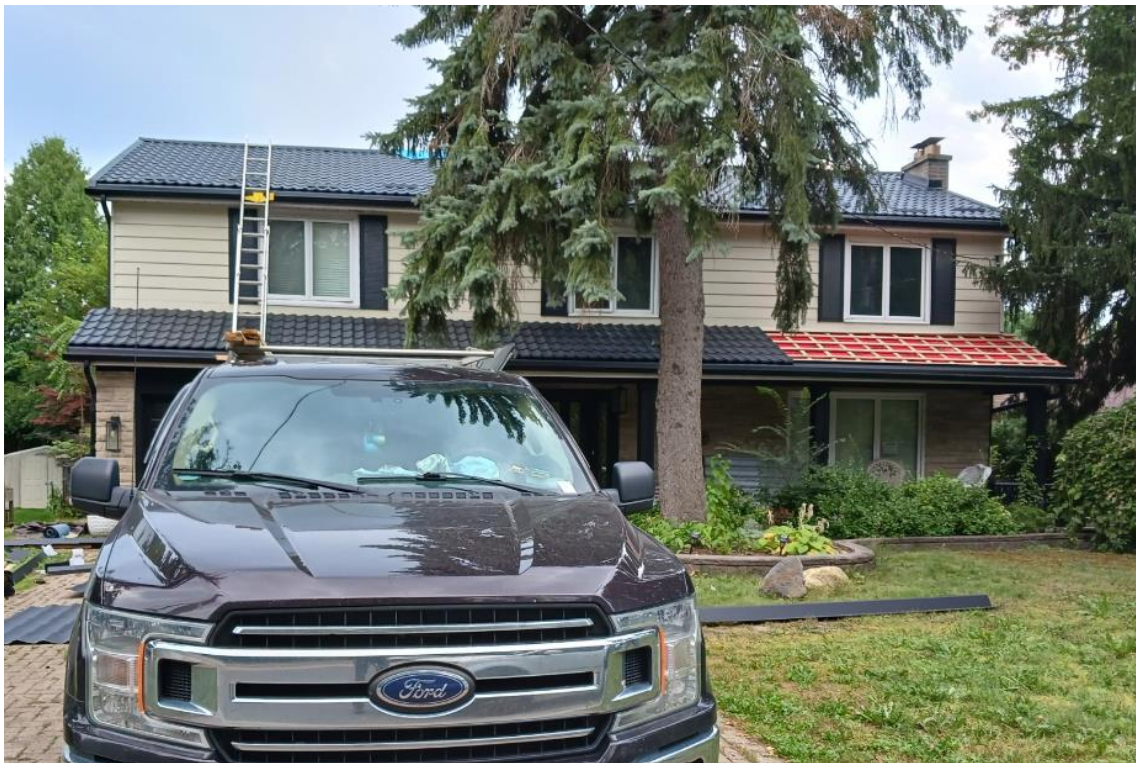
Primary (north) elevation of 146 John Street showing the recently installed roofing material (Source: City of Markham c.2024)
