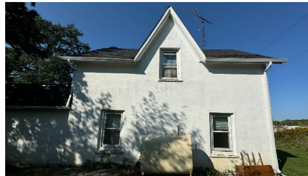
Original Section Of Farmhouse & Original East (Front) Façade With Bricked Over Front Entrance and Peaked Dormer
