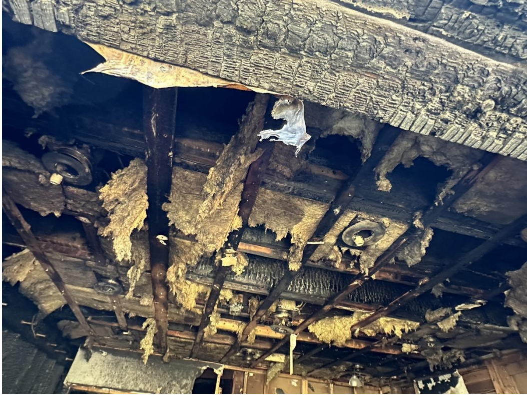
Photo 7 – View of Significantly Charred Joists Above Main Floor
