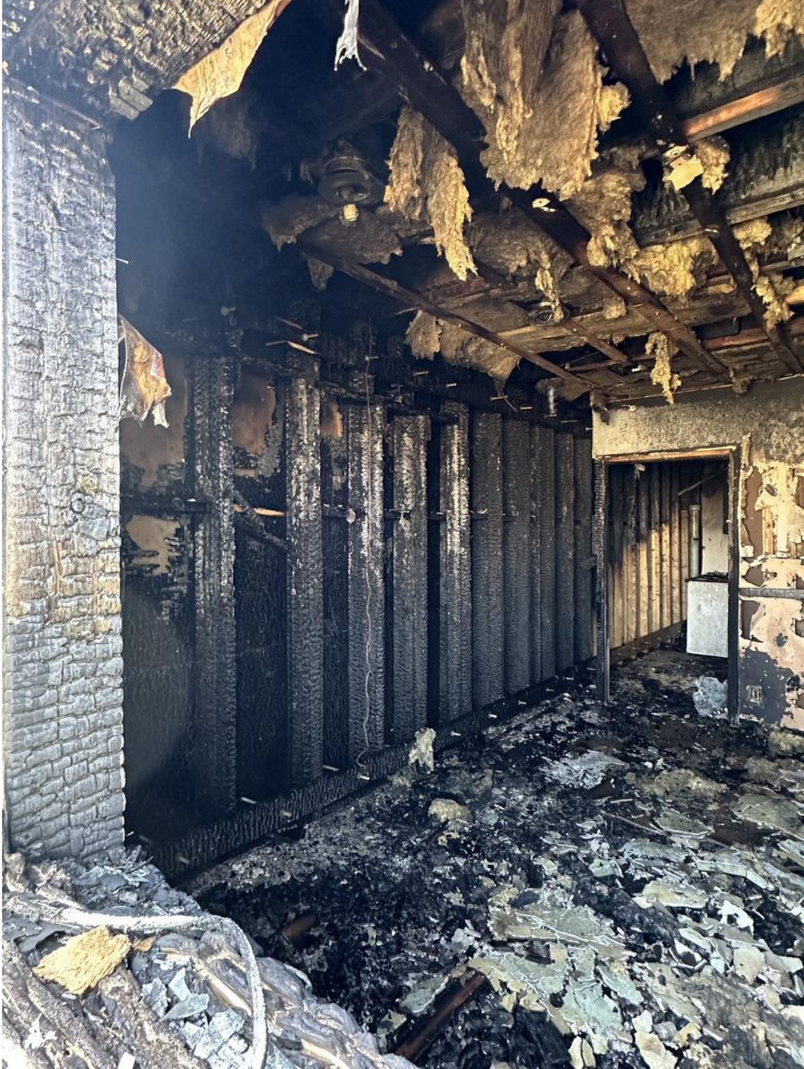
Photo 5 – Interior View Showing Significantly Charred Wall Studs
