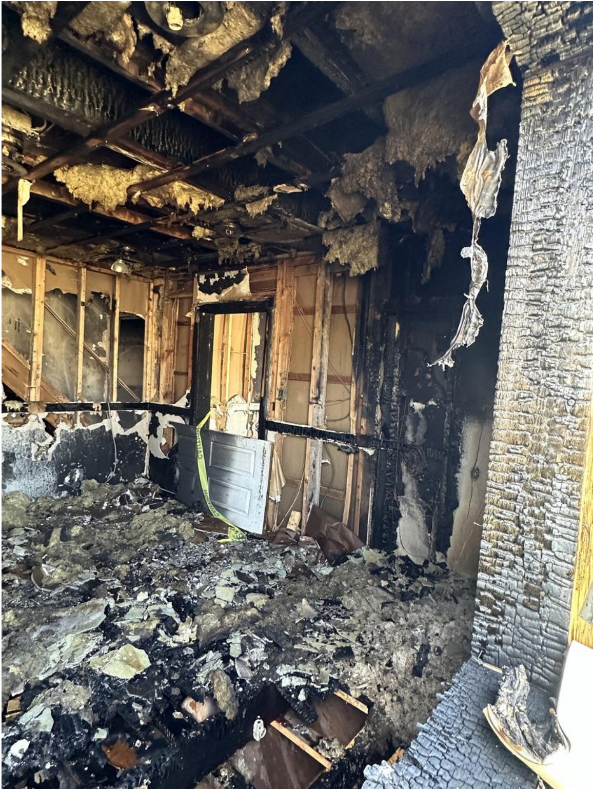
Photo 6 – Interior View Showing Damage to Floor Structure Above and Below Main Floor
