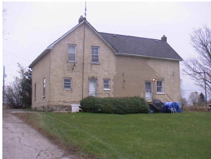
Rear or west view of 10982 Highway 48 showing patch in the brickwork, a possible indication that a rear wing has been removed.
