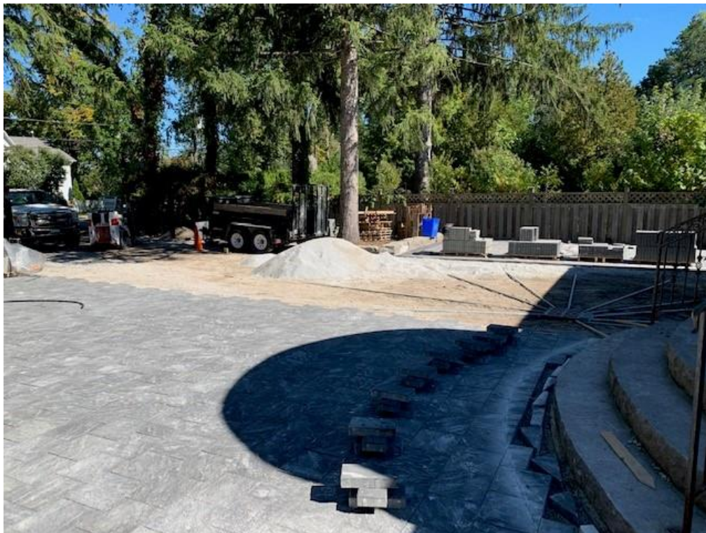
Images of the subject property post-alteration showing the paving of the former lawn (above) and grading work in preparation for the new driveway (Source: City of Markham)
