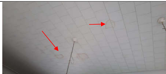
Photo 6: Water staining at the building interior.
