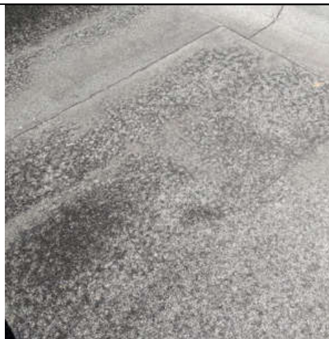
Photo 8: Roofing membrane degranulation. Granules protect roof from UV degradation.
