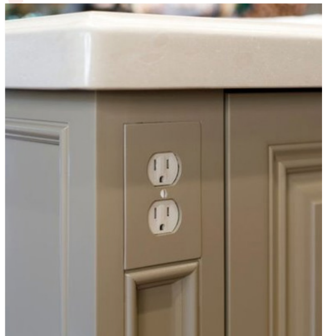
Figure 110. Electrical outlets and light switches at mid-level heights provide the most flexibility over time.
