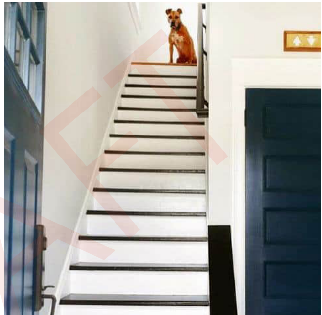
Figure 114. This straight flight of stairs shows how high contrast nosing on the steps can improve safety for some older adults with reduced eye-sight or limited depth perception.
