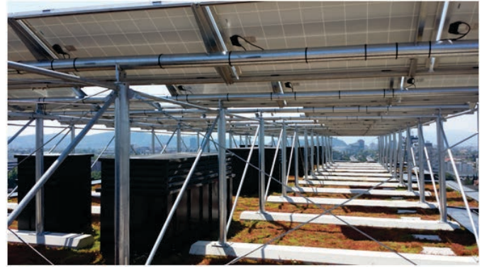
Figure 70: Photovoltaic Panel Array
