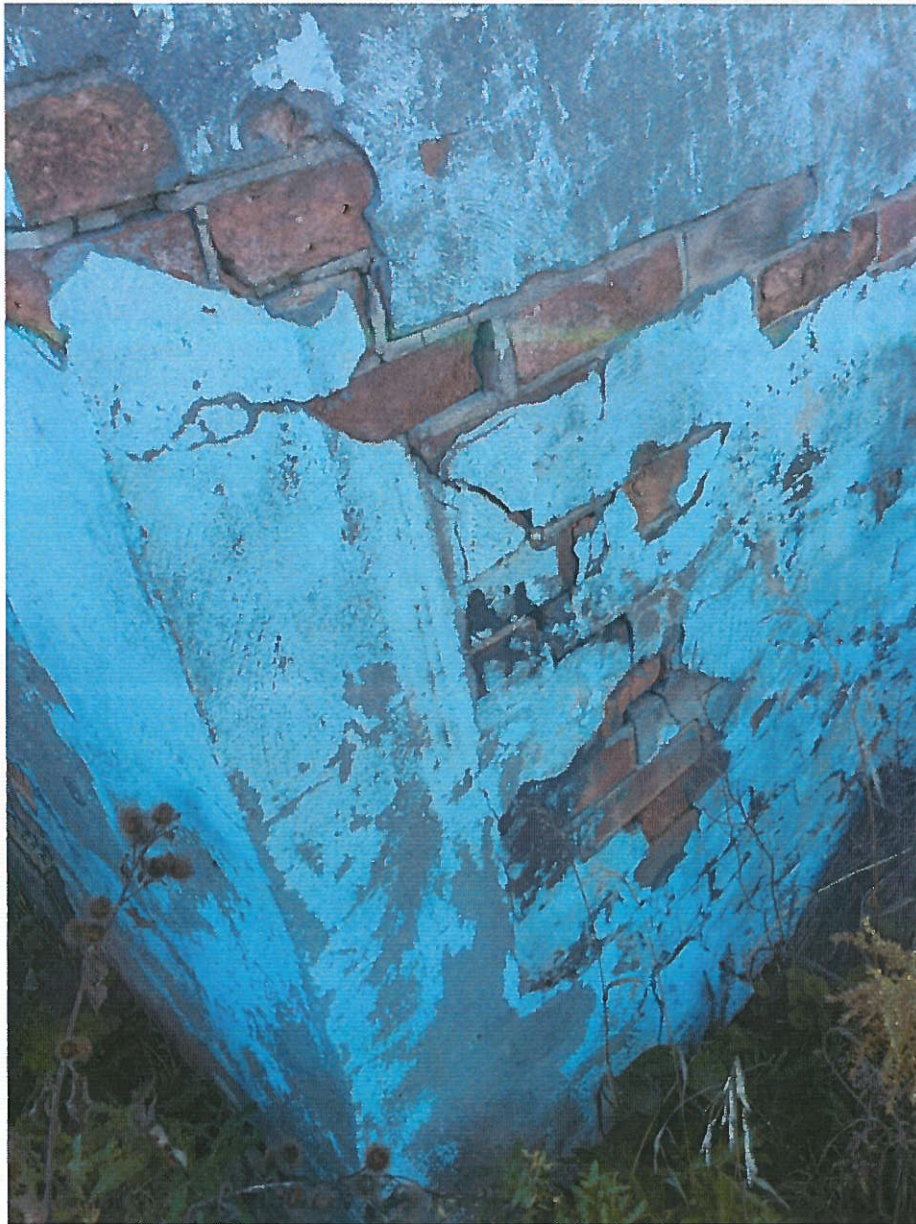
Typical cracking at corners
