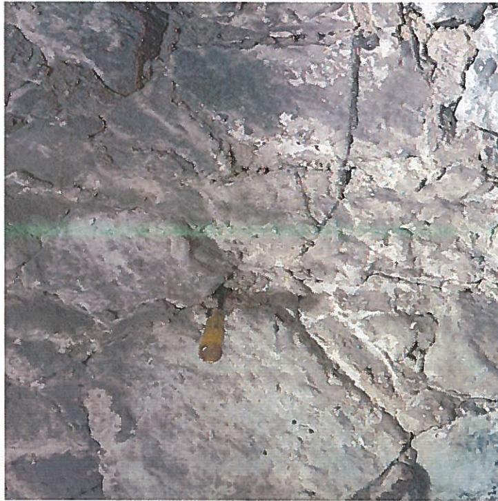
Foundation wall in basement (Screwdriver through mortar)
