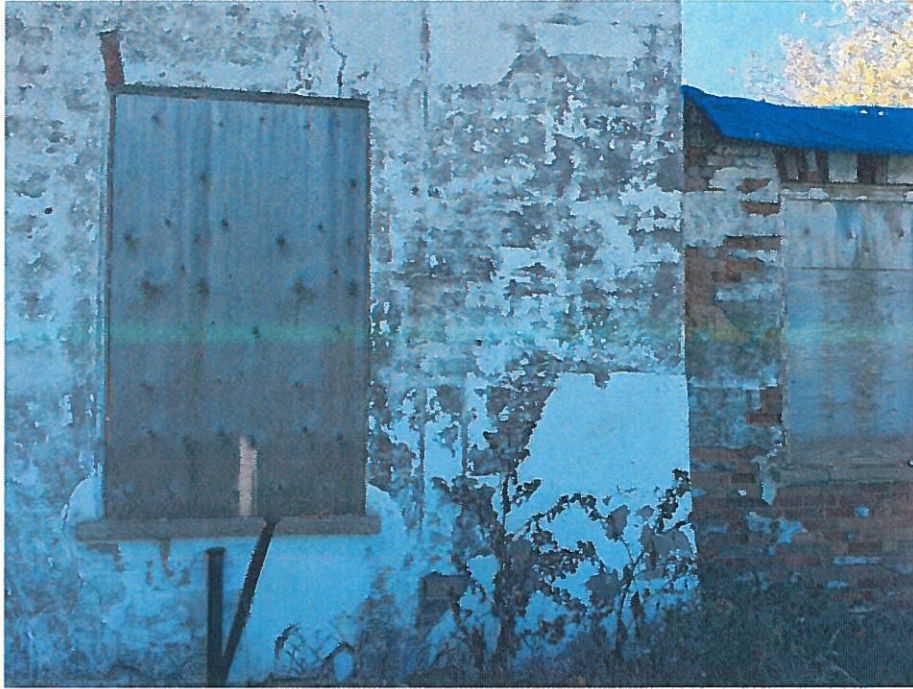
Typical cracking at corners
