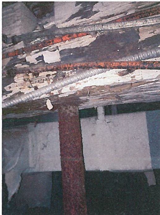
Steel post crushing into beam (no footing can be seen)
