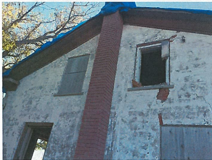
Exterior wall cracking at lintels
