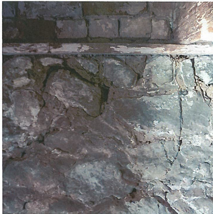
Deterioration of basement wall
