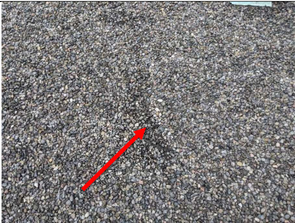
Photo 5: Membrane blister, potential location for future leak.
