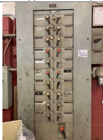
Electrical disconnect switch
