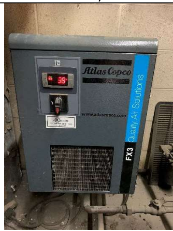
Fire bay pneumatic compressor air dryer
