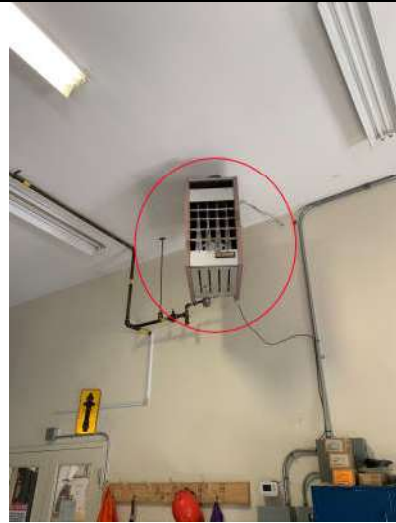
North shop heater
