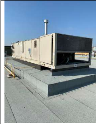
Air handling unit
