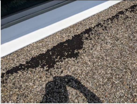
Photo 3: Membrane blueberries, indicative of an older roof.
