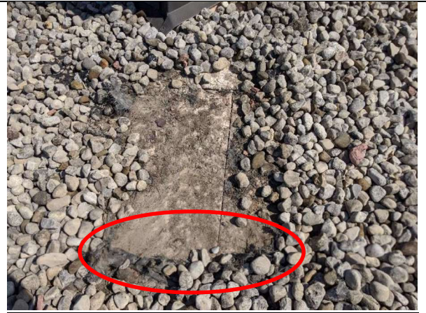
Photo 4: Ballast reducing sheet (black material) deteriorated, should be sandwiched between the ballast (stones) and insulation (Pink material).
