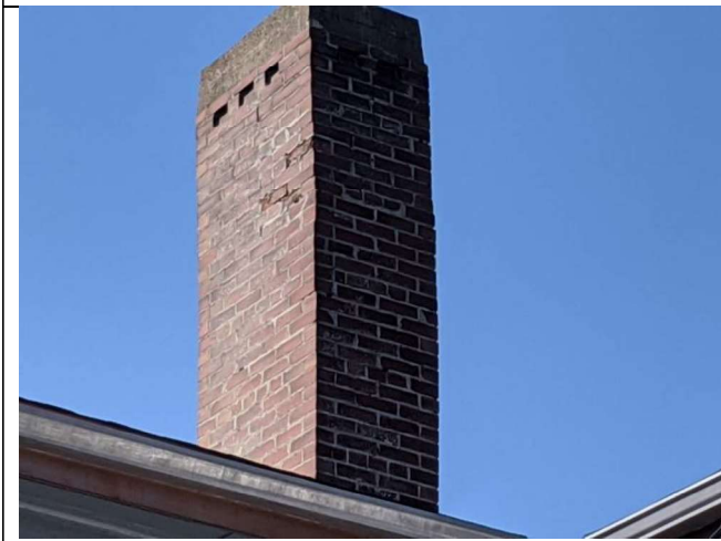
Photo 3: Brick spalls at smaller chimney.
