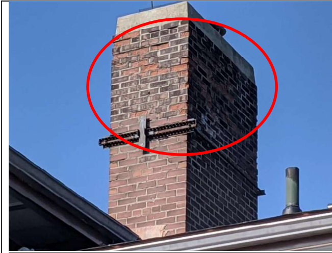
Photo 1: Brick spalls at the larger chimney.
