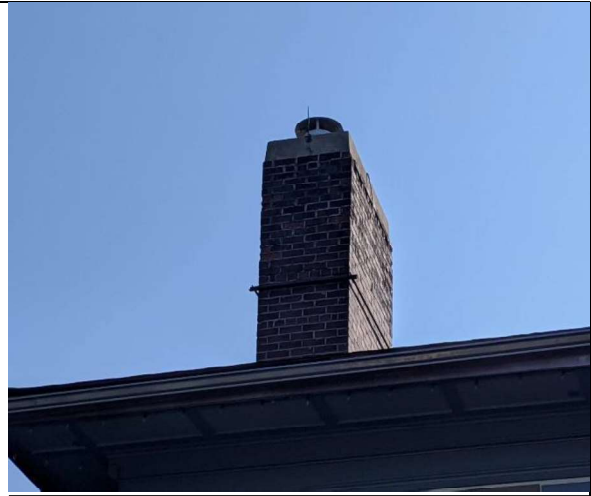
Photo 2: View of the larger chimney from the opposite direction, structural support installed at the chimney.
