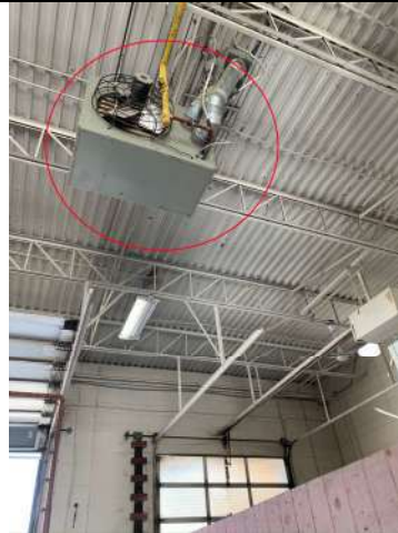
Vehicle wash bay heater
