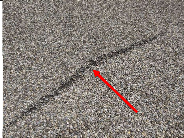
Photo 4: Membrane ridge, potential location for future leak.
