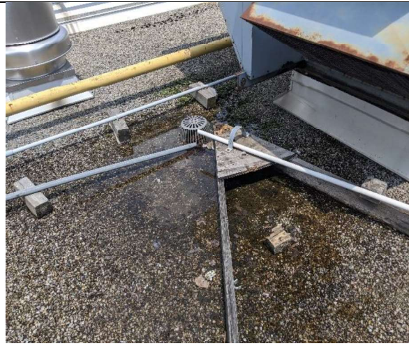
Photo 2: Water ponding on the roof.
