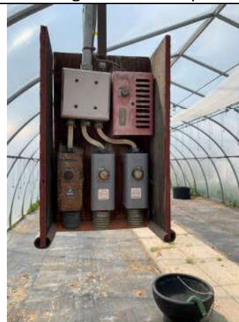
Northeast greenhouse thermostat
