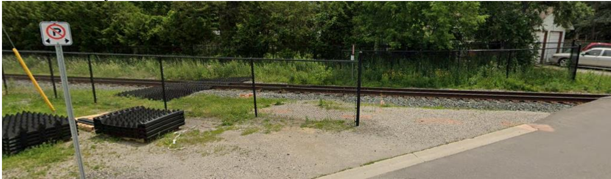
Black Chain Link Fencing used along the railway corridor for safety reasons Eureka Street adjacent to Stiver Mill
