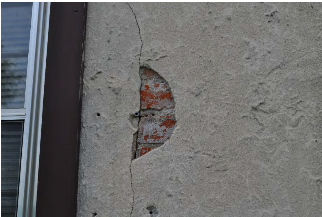
Photo 5: Detail of visible brick structure below cracking stucco
