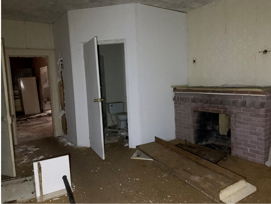
Figure 24: View of first floor, including fireplace (looking west towards kitchen and southern addition) (CU 2020).
