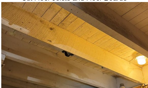
Cut Floor Joists and Floor Boards
