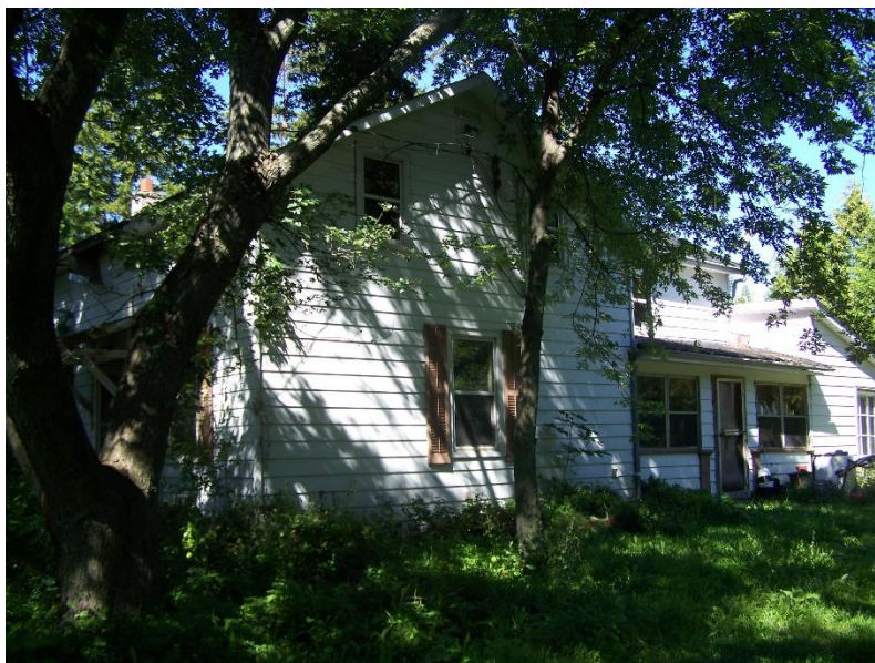
East side view of 11288 Kennedy Road showing rear wing, enclosed porch and shed-roofed addition.
