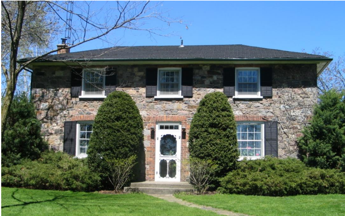
Attachment B- Photograph of Graham-Hallman House Prior to installation of metal roof 2004
