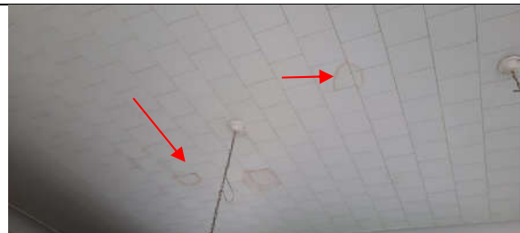
Photo 6: Water staining at the building interior.
