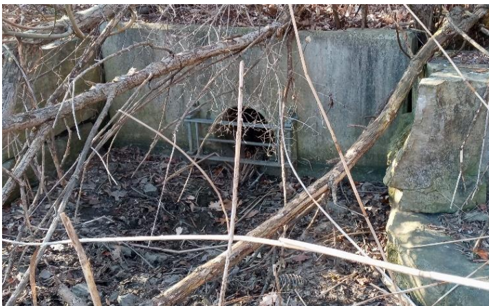
East Pond –Inlet from South Splitter (April 2022)
