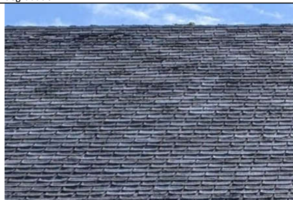
Photo 3: Widespread curling of the roofing shingles. Roof has failed.
