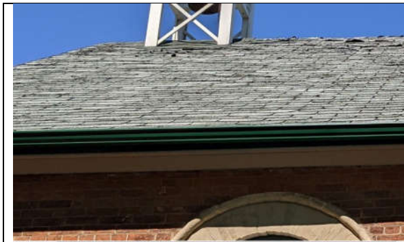
Photo 1: Roof shingles are curling at west elevation. Sign of UV degradation.
