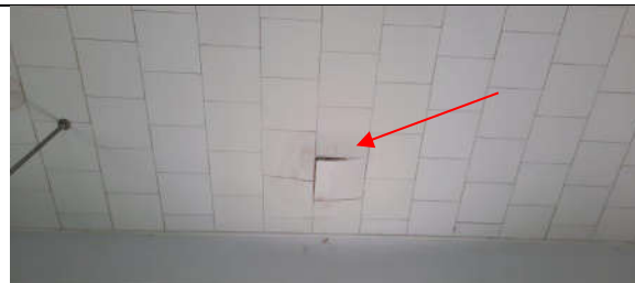
Photo 5: Leaking at building interior, significant leak event to cause this "bubbling" of the tile.
