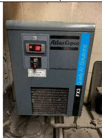
Fire bay pneumatic compressor air dryer
