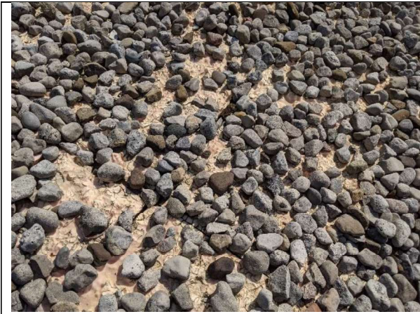
Photo 1: Deteriorated insulation beneath ballast (stones).
