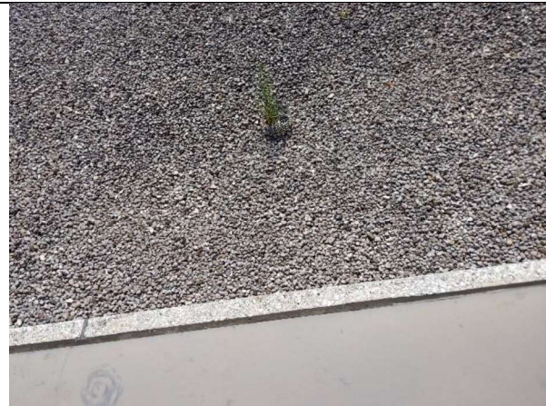
Photo 2: Vegetation on roof indicative of roof poor drainage.
