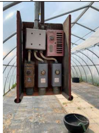
Northeast greenhouse thermostat
