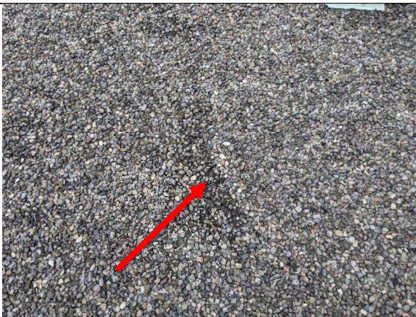
Photo 5: Membrane blister, potential location for future leak.
