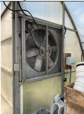
Northeast greenhouse circulating fan
