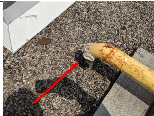
Photo 6: Sealant Deterioration at gas line penetration.
