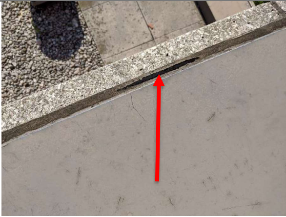
Photo 3: Split in the sealant between the precast panels and metal flashing.
