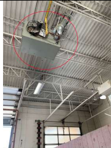
Vehicle wash bay heater
