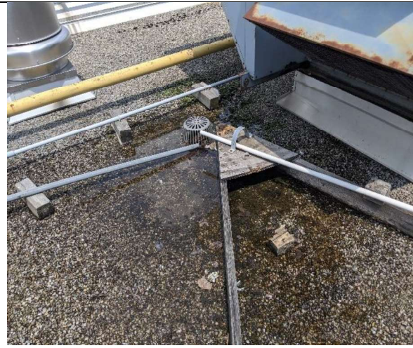
Photo 2: Water ponding on the roof.
