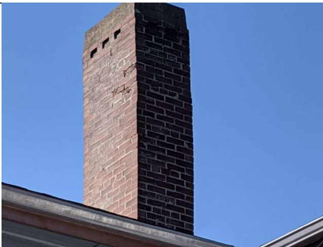
Photo 3: Brick spalls at smaller chimney.
