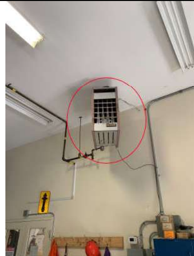
North shop heater
