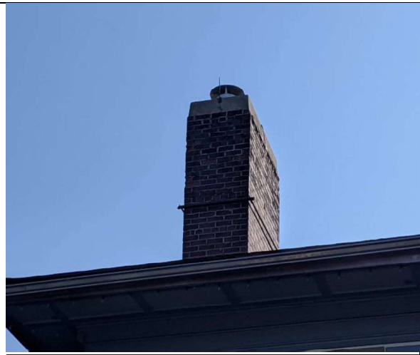
Photo 2: View of the larger chimney from the opposite direction, structural support installed at the chimney.
