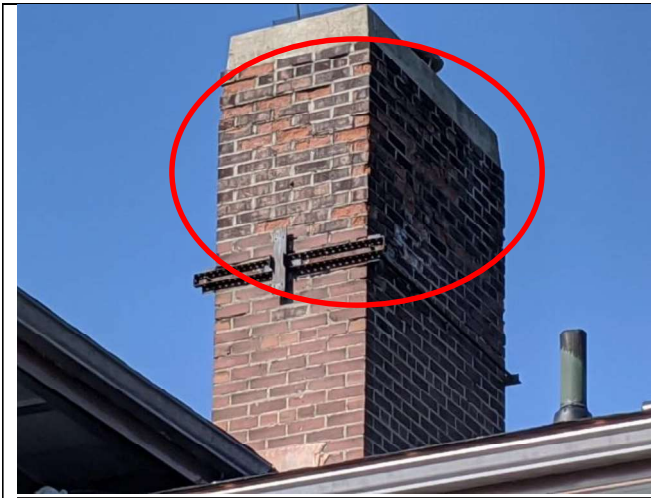
Photo 1: Brick spalls at the larger chimney.
