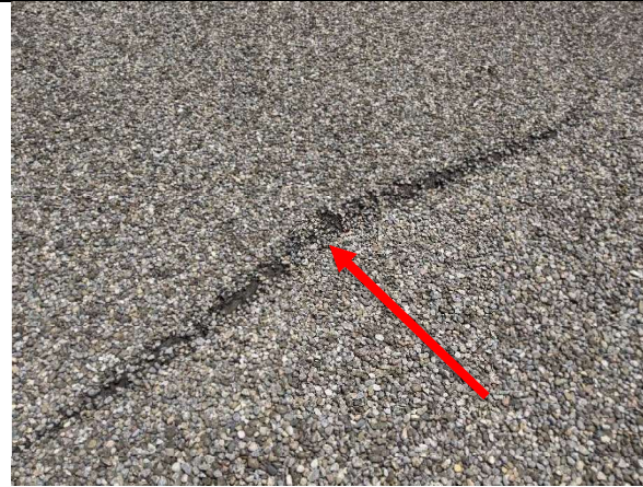
Photo 4: Membrane ridge, potential location for future leak.
