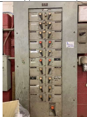
Electrical disconnect switch
