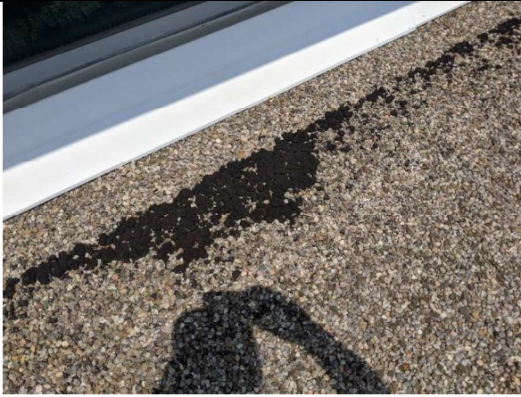
Photo 3: Membrane blueberries, indicative of an older roof.
