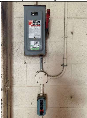
Garage door disconnect
