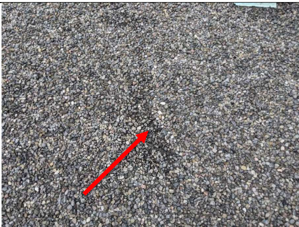
Photo 5: Membrane blister, potential location for future leak.
