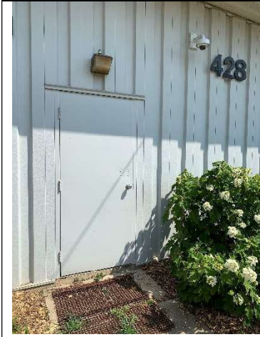
Painted metal door with frame
