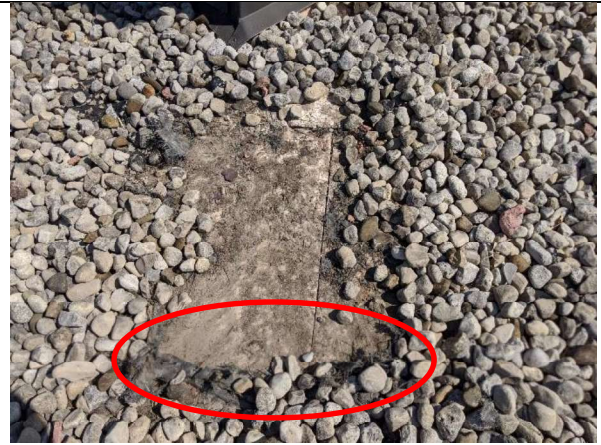
Photo 4: Ballast reducing sheet (black material) deteriorated, should be sandwiched between the ballast (stones) and insulation (Pink material).
