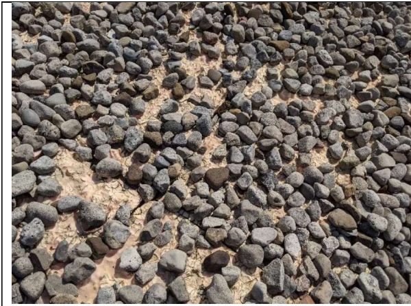
Photo 1: Deteriorated insulation beneath ballast (stones).
