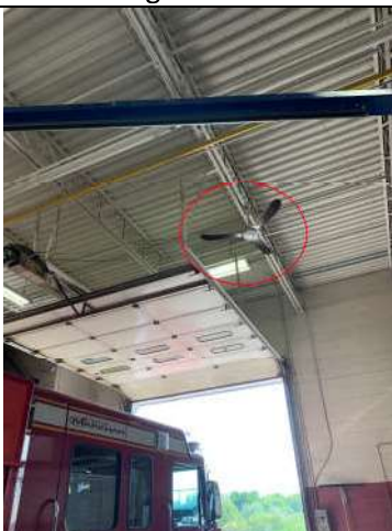
Fire bay circulating fans
