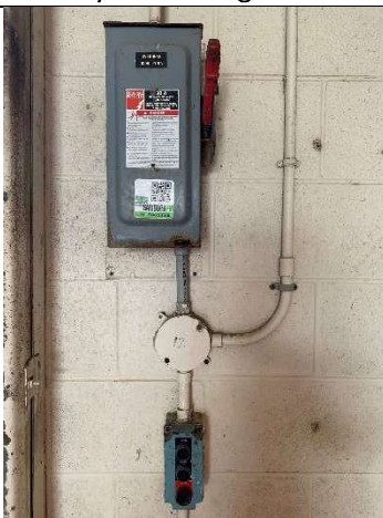
Garage door disconnect
