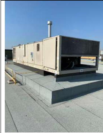
Air handling unit
