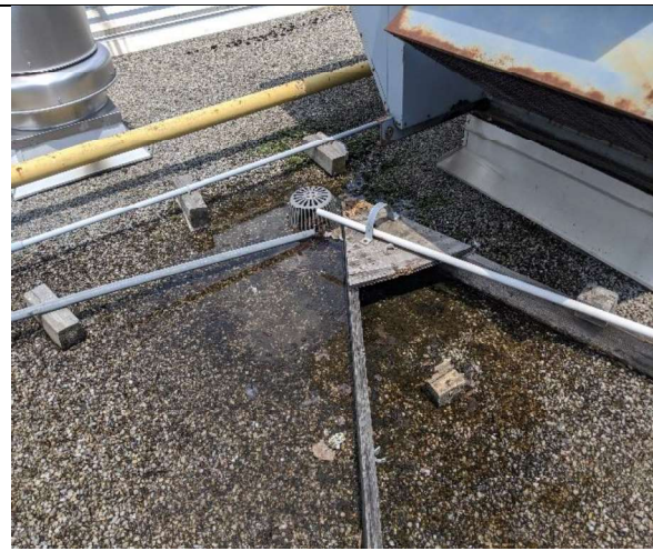
Photo 2: Water ponding on the roof.
