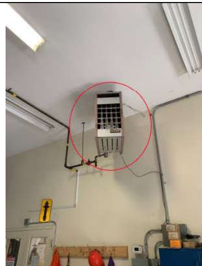
North shop heater
