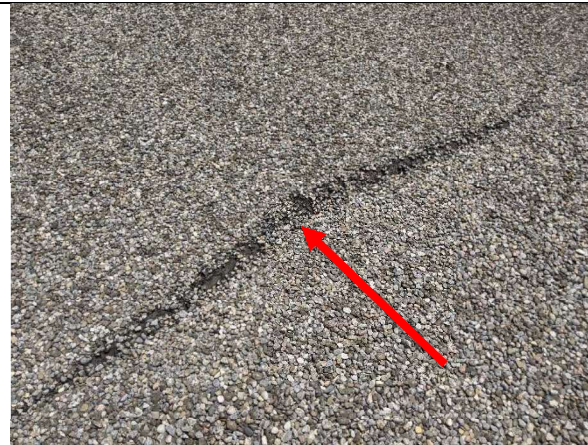
Photo 4: Membrane ridge, potential location for future leak.
