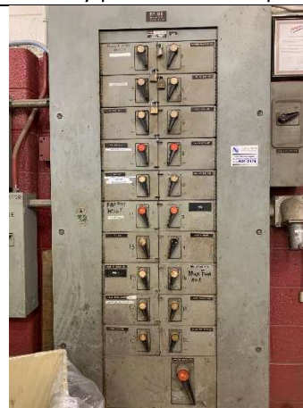
Electrical disconnect switch
