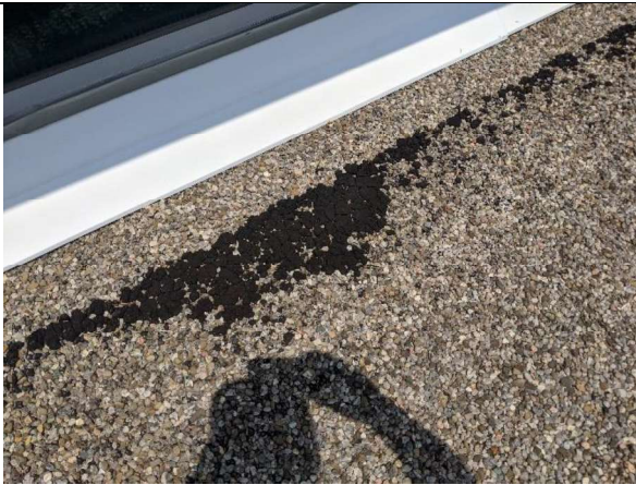
Photo 3: Membrane blueberries, indicative of an older roof.
